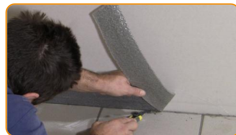
When the flooring application is completed, cut the exceeding part of the edging strips.
