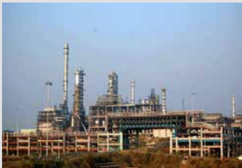
Bharat Oman Refinery, Bina, India
