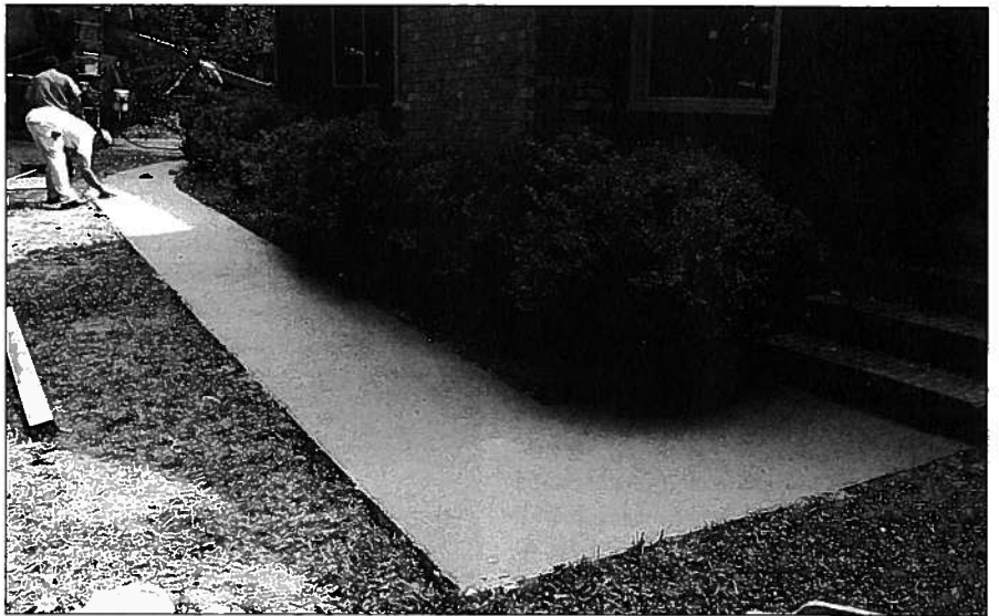
This walkway with re-entrant corner at one end and a curve at the other with no joints remains crack-free after more than three and a half years.
